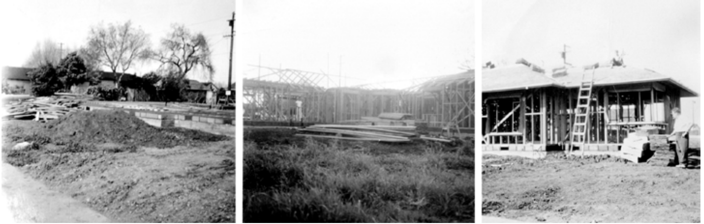
House construction at 1991 Webster Street in 1949 started in February and finished in August
